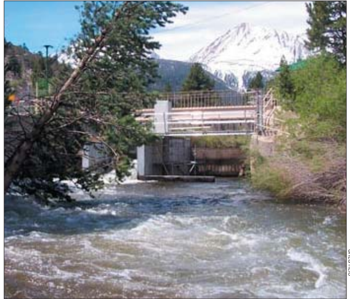
The upgraded Lee Vining Creek sediment bypass facility no longer blocks sediment needed for fish habitat and new vegetation, but allows it to pass downstream.
