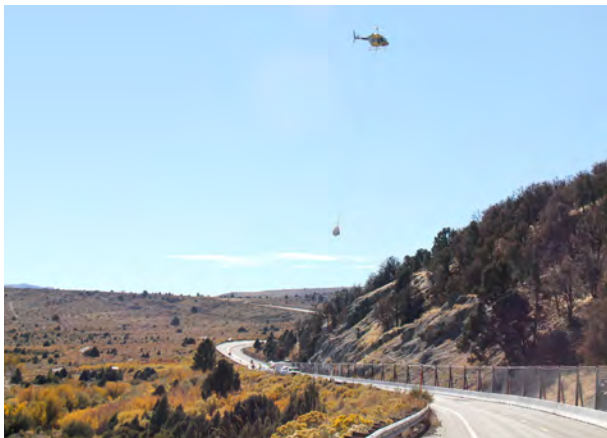
The Committee successfully advocated for special erosion control methods in the Lee Vining Rockfall Safety Project.
