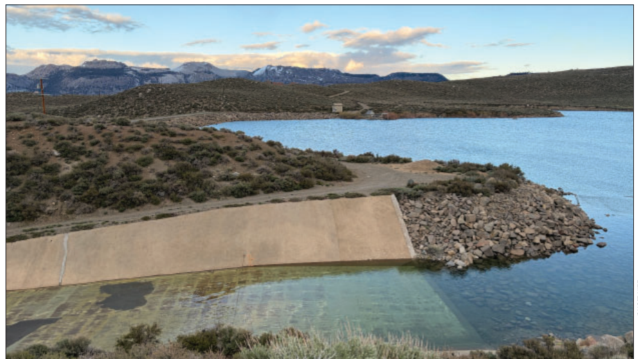
DWP submitted the Grant Lake Reservoir Dam Project work plan to state regulators this spring. Most of the project is necessary to repair aging infrastructure.
